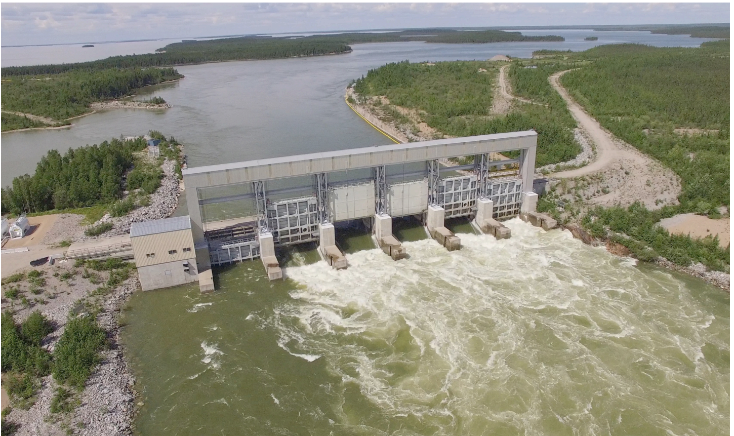
The Missi Falls Control Structure during a sudden and extreme release of water down the Lower Churchill, June 2020. Photo courtesy of Michael Tyas / Wa Ni Ska Tan
