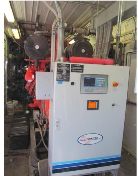
Photo: This picture of a biogas generator room was taken during the committee's visit to Mr. Laforge's farm in St. André, New Brunswick, in November 2012.
