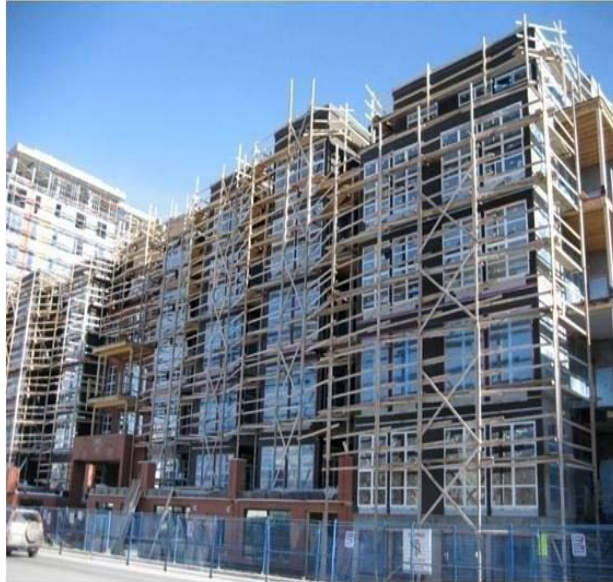
Figure 4 – Ellis Building, Kelowna, B.C., under construction – British Columbia’s first six-storey wood-frame building 47
